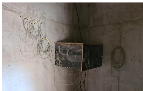
Figure 52. Box containing data acquisition equipment
