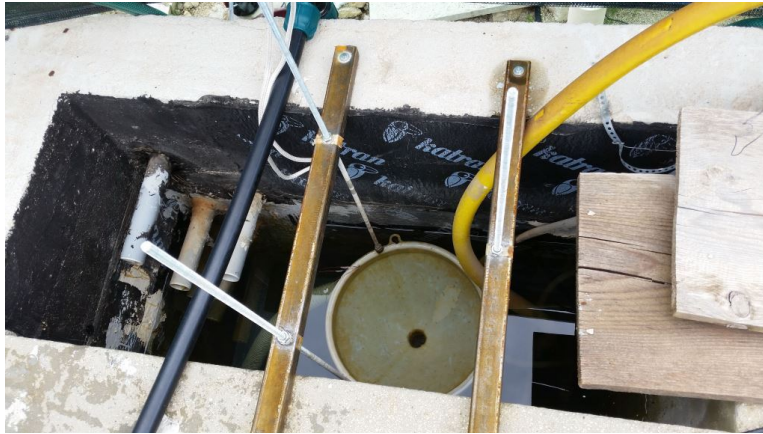
FIGURE A.17: Overflow in downstream reservoir.
