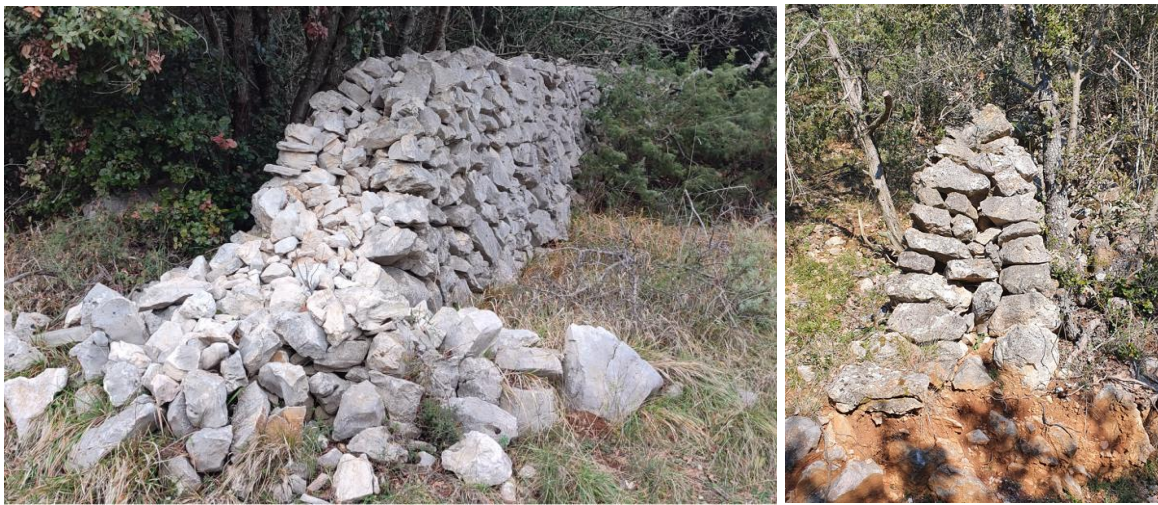
Figure 15. A cross-section of the double wall a) close to Pukonjina (2021) and b) close to Stanić (2021)
